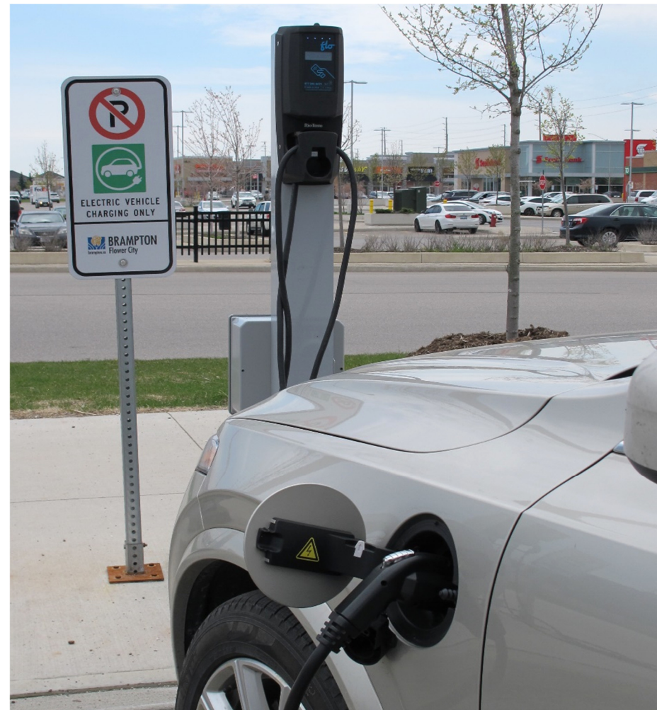
EV charger at Springdale Library
