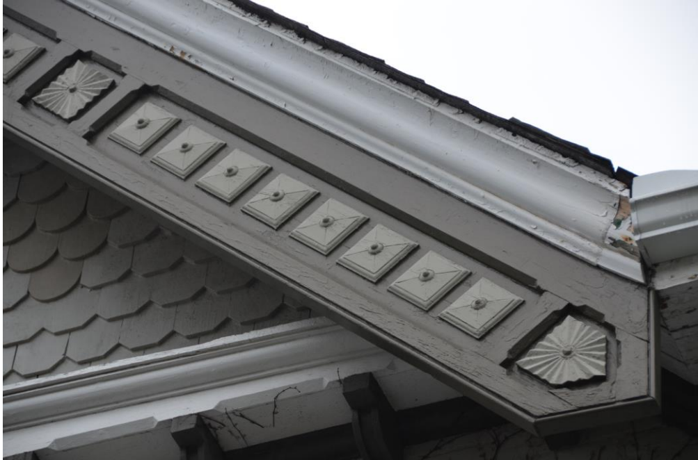
Figure 8: Vergeboard detailing on front façade and detailed shingles (Source: City of Brampton, 2019)
