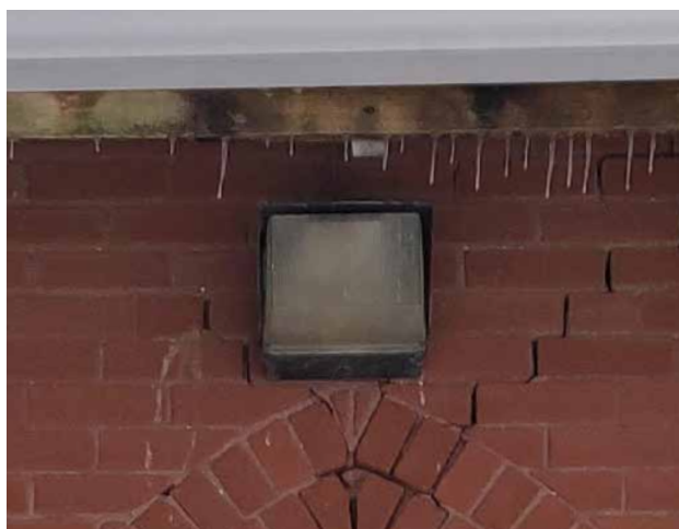
Fig. 2.43. Exterior lighting fixture to be removed.
