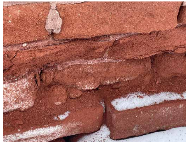
Fig. 2.4. General condition of brick near grade.
