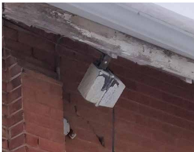
Fig. 2.42. Exterior lighting fixture to be removed.
