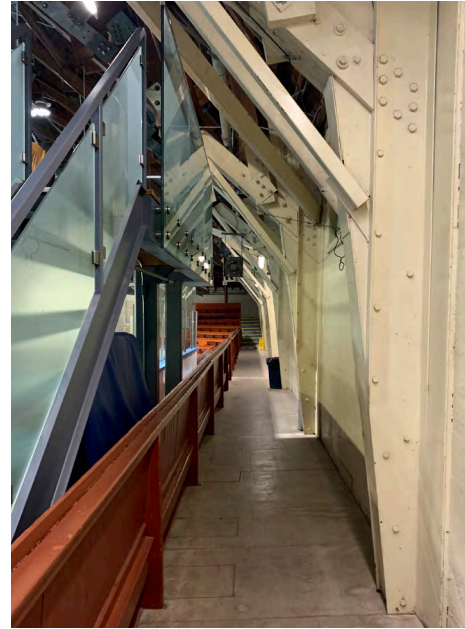
View of interior where new addition is to be located Source: ATA Architects, 2022
