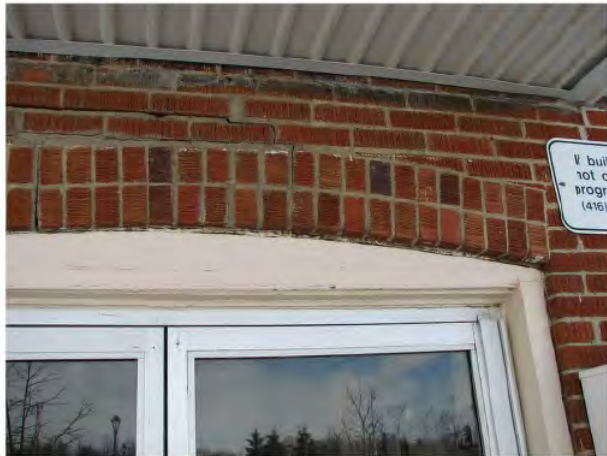
Detail showing portion of masonry wall on front façade. This image shows the brick arch of the east entrance. Note step crack. Masonry repairs are required.
