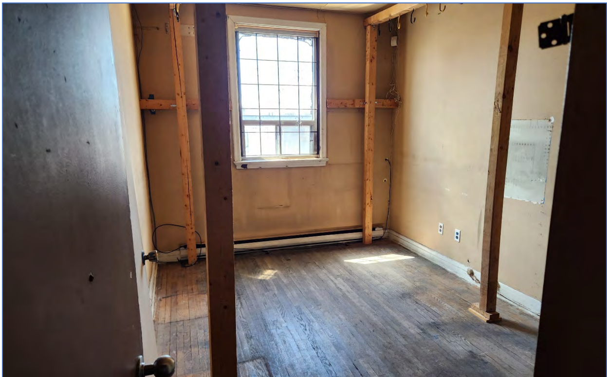
Photo 70: View southwest showing the bedroom/office with a wood floor in the east suite
