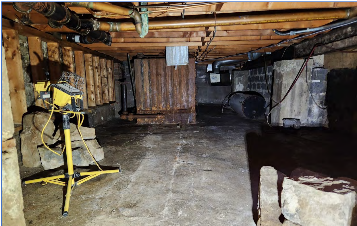
Photo 74: View northeast showing the boiler
