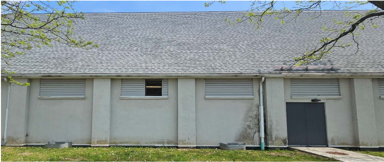
Fig. 4.2: Existing 36" x 36" Intake Louvre to be relocated to next bay left. Source: +VG Architects
