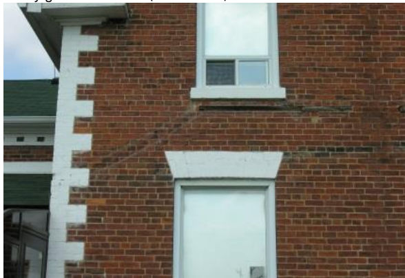
Figure 38 South wall, detail showing exposed wood plate at second floor window sill and "staircase crack."
