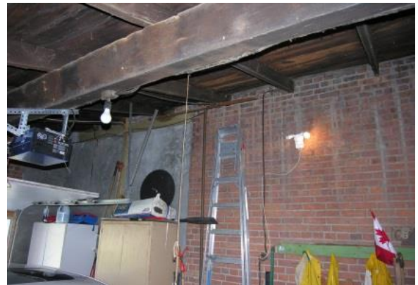
Figure 39 Garage interior showing difference in wall materials of the various additions and alterations.
