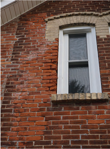
Detail view of deterioration, weathered brick at window edge.
