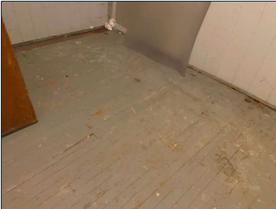
Photograph 6: Water damage to floor finishes
