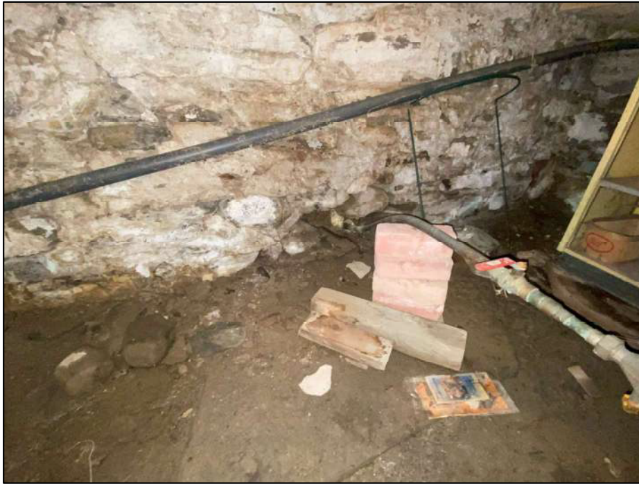
Photograph 4: Undermined section of foundation wall
