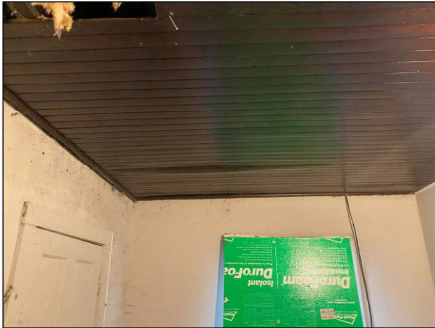
Photograph 5: Water damage to ceiling finishes
