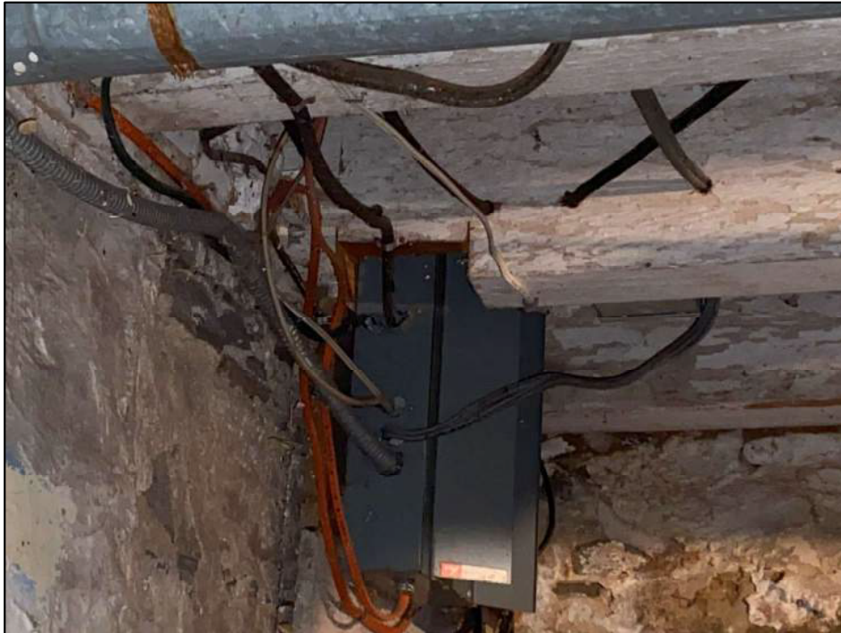
Photograph 3: Notched joist behind furnace
