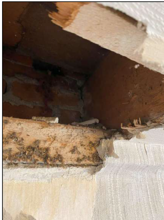
Photograph 2: Section of removed ceiling finishes at the middle of the south wall
