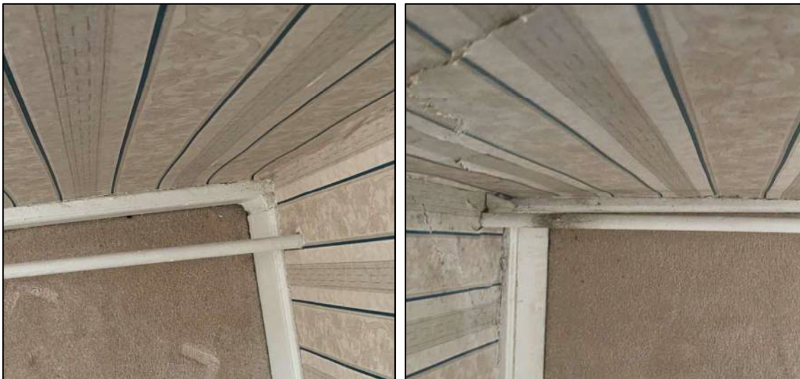
Photograph 1a & b: Relative deflection of wall based on offset from tension rod
