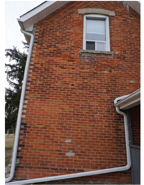
Brick damage along window
