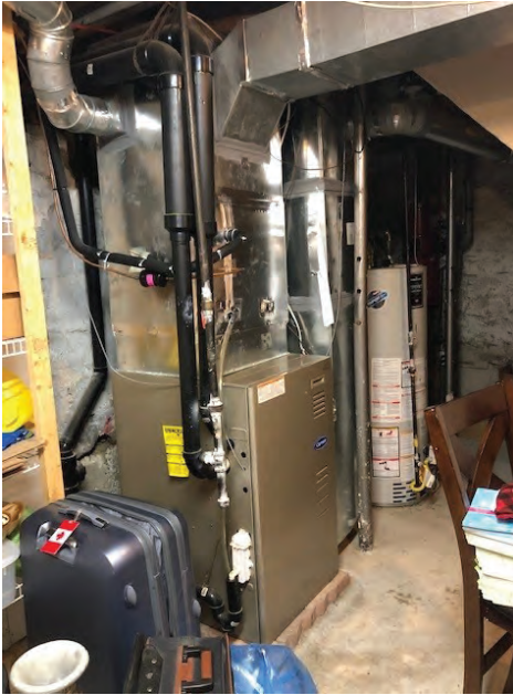
View of furnace and boiler, located in basement Source: ATA Architects Inc. 2021
