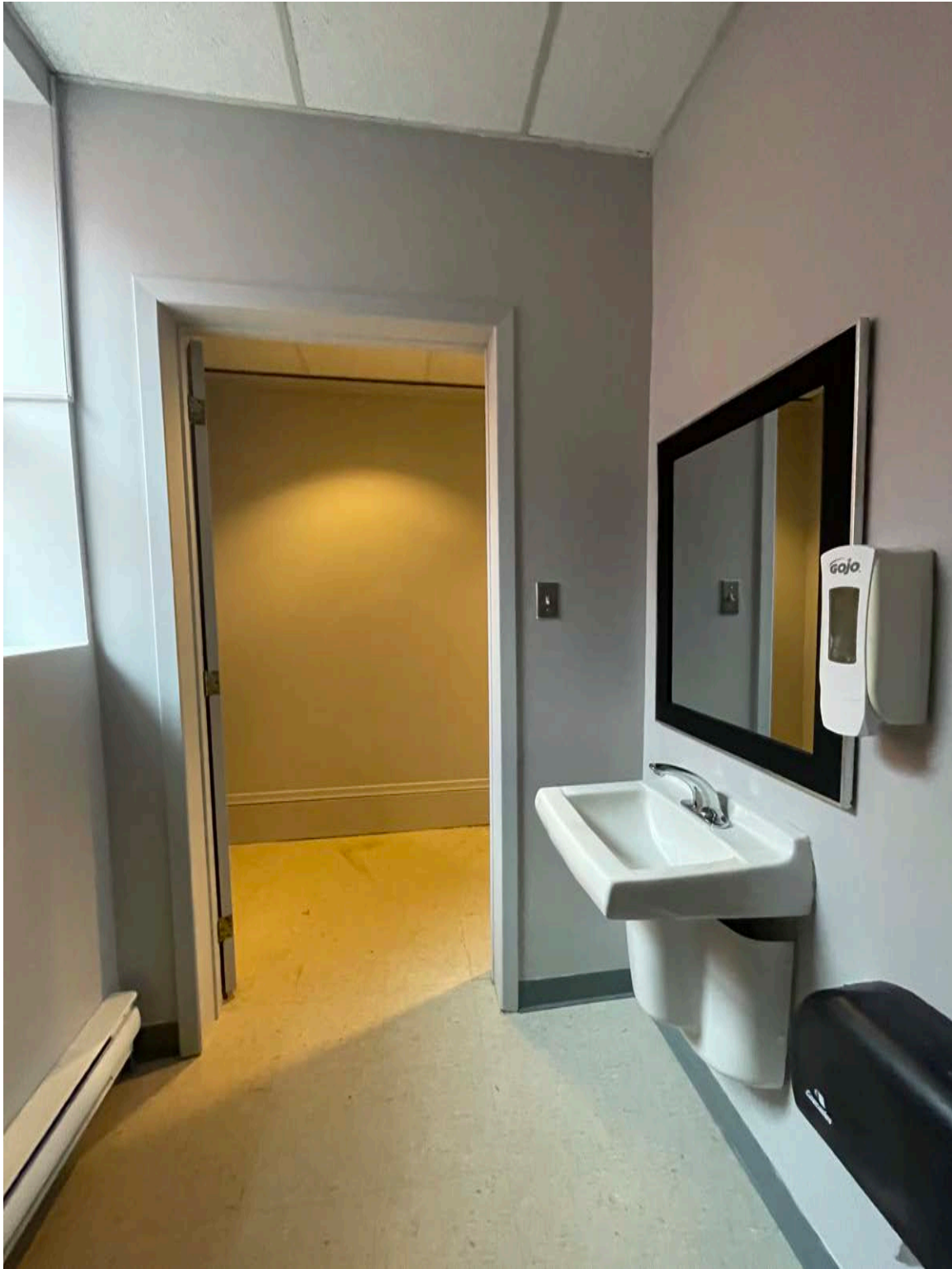
WASHROOM – existing two-piece washroom on the lower level – nor original features or finishes - modern fixtures, drywall, vinyl flooring & acoustic tile ceiling – door casing on interior side is not original
