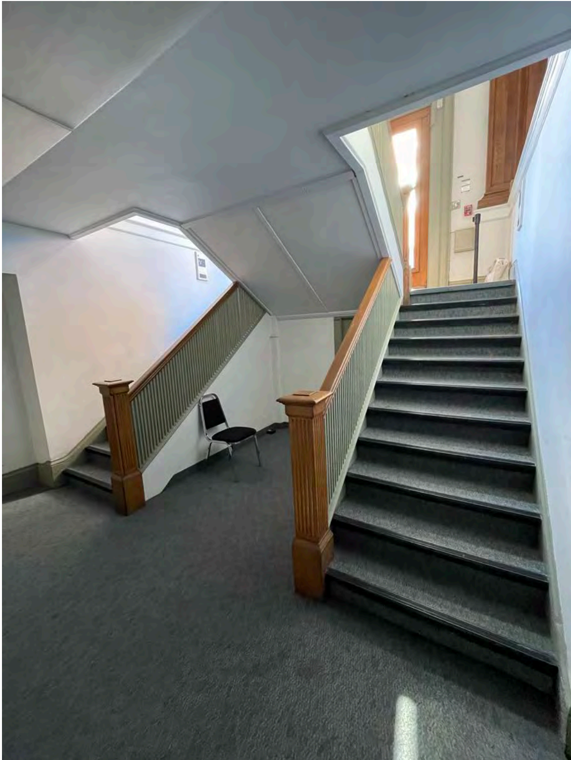
INTERIOR – LOWER LEVEL: view looking up to the entrance vestibule from the lower level – two sets of stairs down to the lower level and one set of stairs to the main floor – original features and finishes include the oak newel posts and railings – plaster & lathe walls and wood baseboards – wall to wall carpet has been installed on the original stair treads and risers
