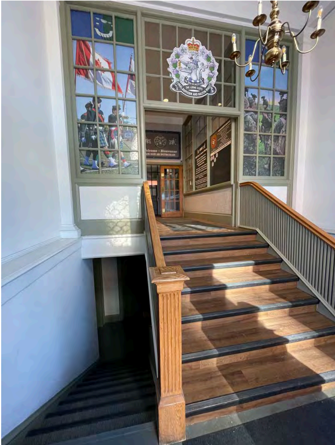
INTERIOR – VESTIBULE: original interior finishes and features include the oak newel posts and railings, the plaster & lathe walls, wood & plaster trim and the glazed partition wall at the top of the stairs – new vinyl flooring and carpeting has been installed on top of the original stair treads and risers
