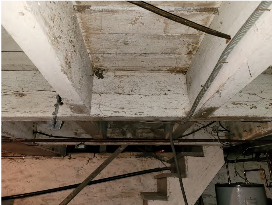
Figure 56: Exposed floor joists left in the rough in the south half of the main block
