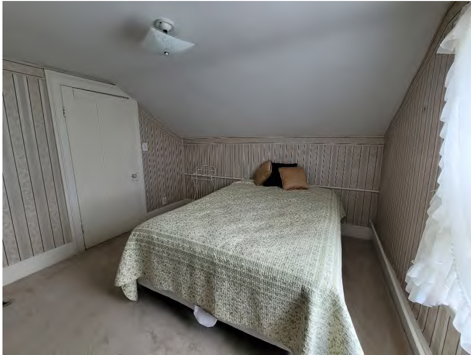
Figure 47: Southeast room with tie rod along east and south walls, facing east
