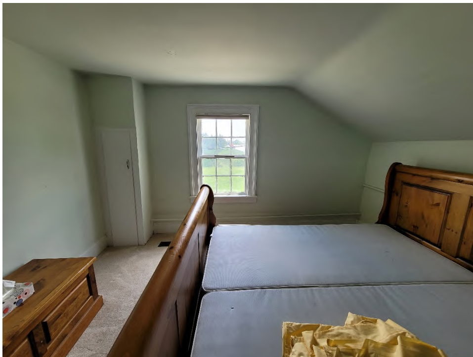
Figure 48: Southwest room with tie rod along south and west walls, facing south
