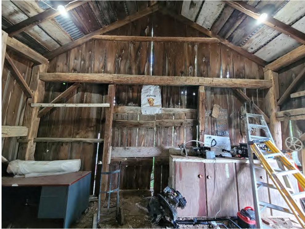
Figure 67: Interior of the driveshed with drop tie-beam, hand-hewn posts and plates and east doorway, facing east
