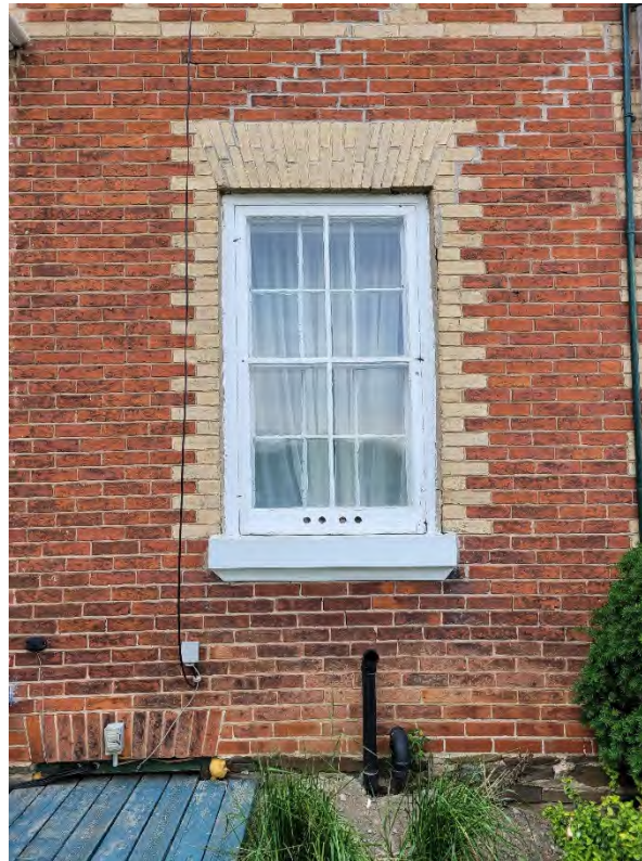
Figure 24: Six-over-six window with wood storm, buff gauged or rubbed brick voussoirs and quoins, and a lug sill with aluminum covering
