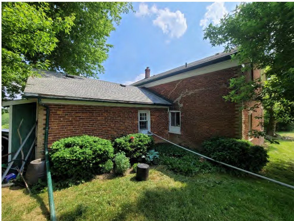
Figure 72: Evidence of cracks on the east facade of the main block.
