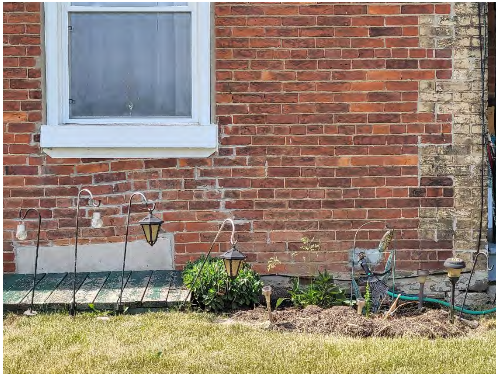
Figure 73: Settlement and movement of load-bearing brick masonry on south end wall
