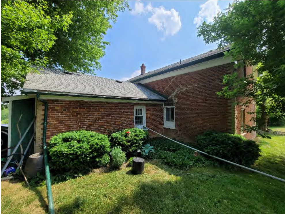
Figure 17: North façade of the rear wing and east façade and north end wall of the main block
