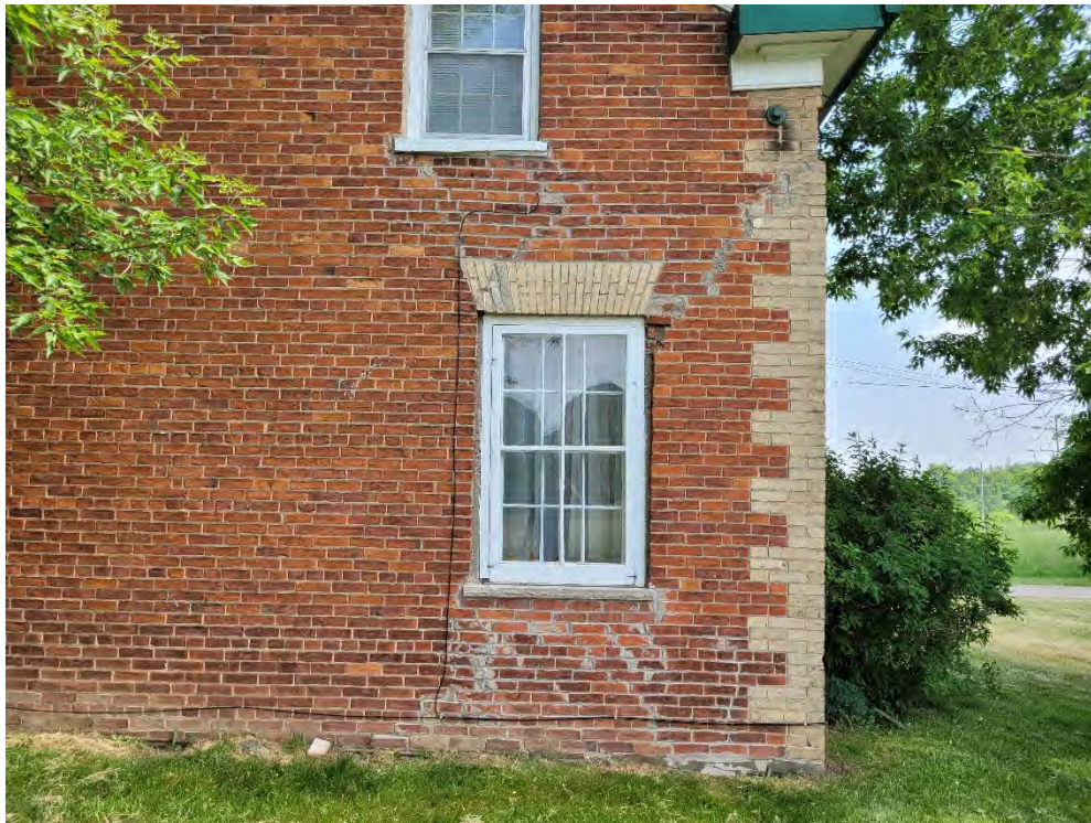
Figure 71: Evidence of cracks radiating from the first level window on the north end wall.
