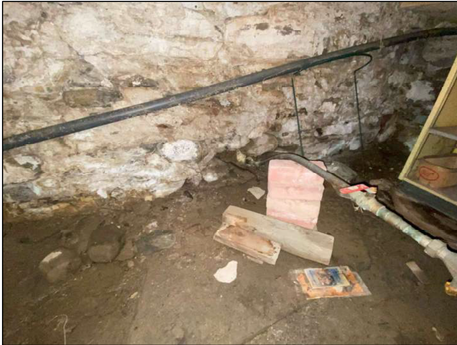
Photograph 4: Undermined section of foundation wall
