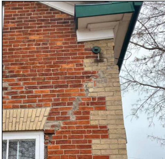
Photograph 7: Cracks and displacement at accent masonry
