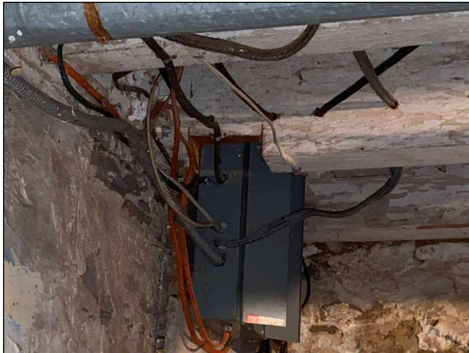
Photograph 3: Notched joist behind furnace
