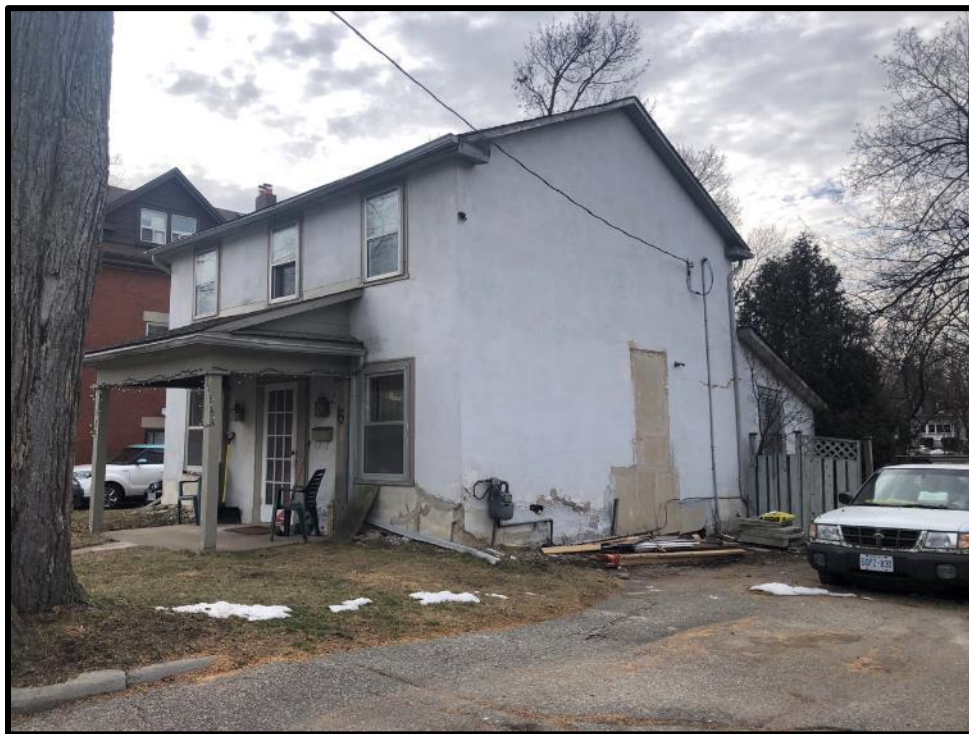
Image 4: Northwest Corner of 15 Isabella Street (Photo taken February 7, 2024; Facing South)
