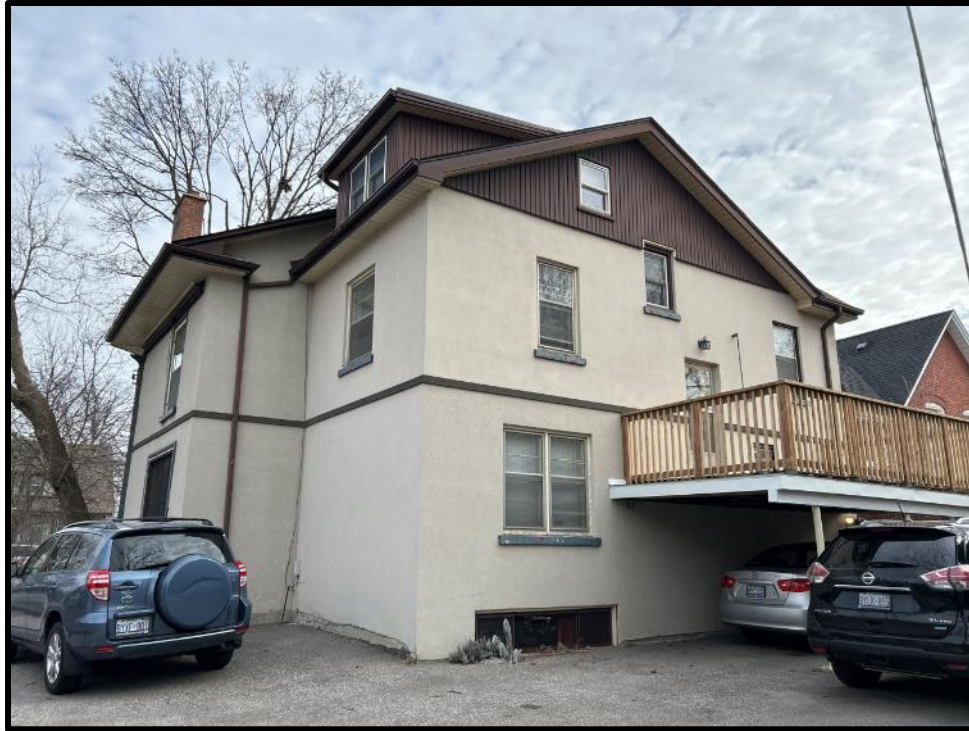
Image 5: Rear (South) Elevation of 227 Main Street North (Photo taken February 7, 2024; Facing East)
