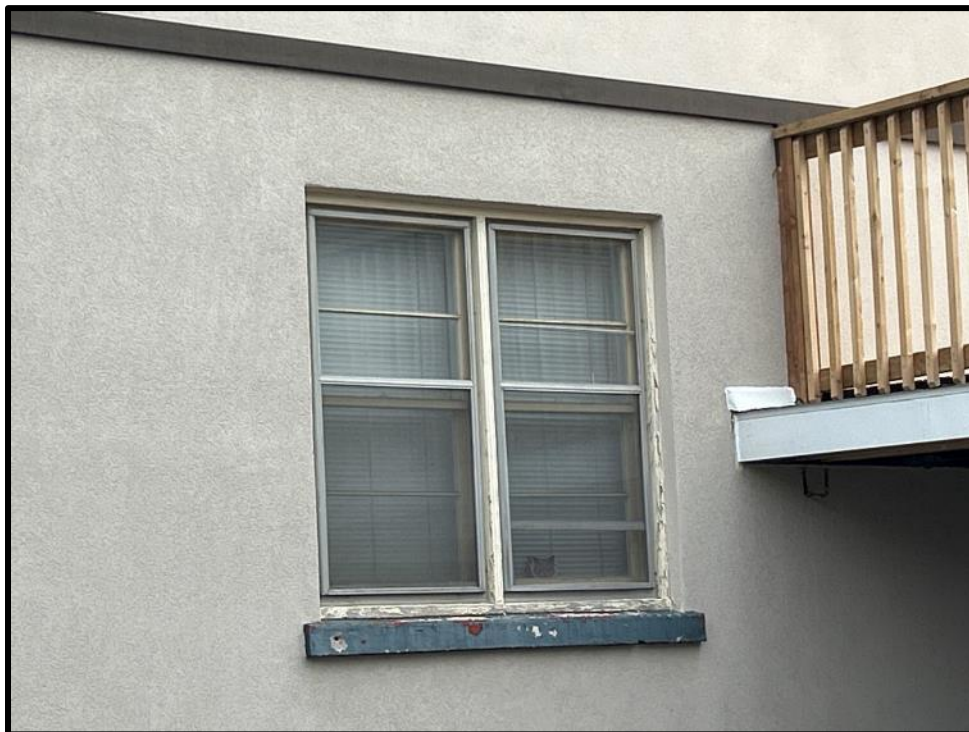
Image 6: Detail of Window Opening on South Elevation of 227 Main Street North (Photo taken February 7, 2024; Facing East)
