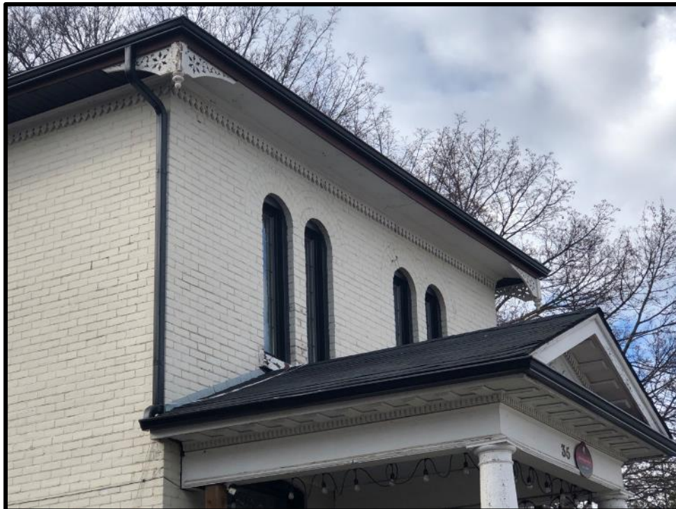
Image 4: Detail of Cornice and Window Openings of 35 Elizabeth Street North (Photo taken February 7, 2024; Facing West)
