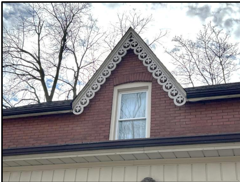
Image 2: Detail of Gable Peak on Façade of 41 Elliott Street (Photo taken February 7, 2024; Facing South)
