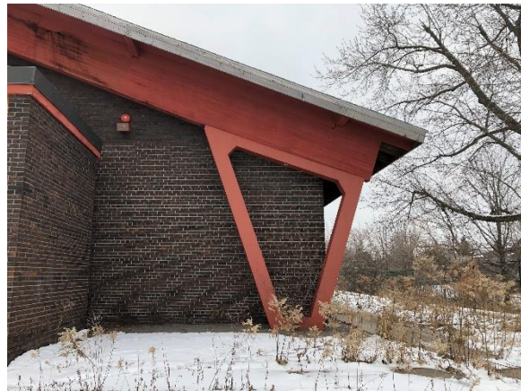
Image 8: View of the concrete pillar supporting the glulam beam, note all concrete pillars are of this shape, but the other concrete pillars are partially enclosed inside the building.
