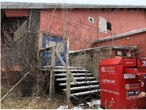
Image 25: View of the stairs and door at the northmost corner of the rear elevation.
