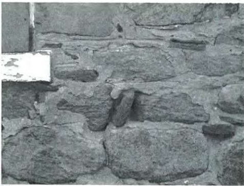
Mortar erosion, west side.
