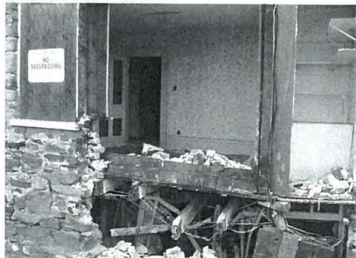
South side. Some interior trim is visible, including wide baseboards and door casing.
