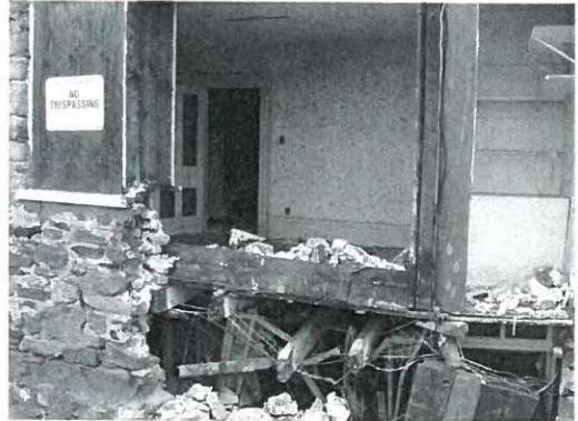
South side. Visible evidence of rot at joist ends.
