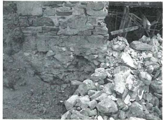
South side. Even material not involved in general failure has fallen away.
