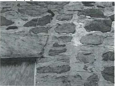
Crack propogation south side.
