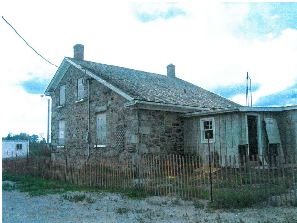
Figure 15: South and east façades of Breadner House prior to demolition (Source: City of Brampton 2009)
