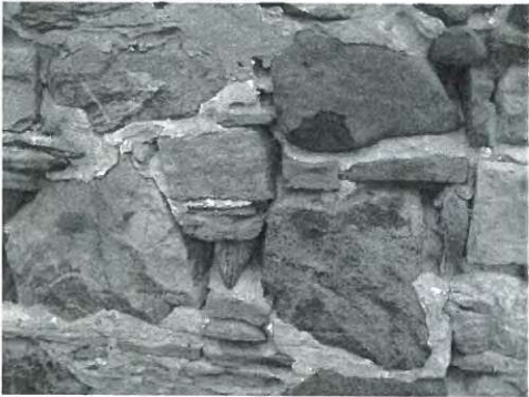
Mortar erosion, west side.
