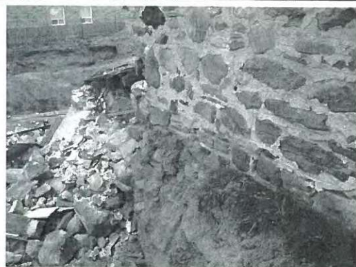
North side foundation, where salt-box joined. Even the intact foundation appears to be unconsolidated rubble.
