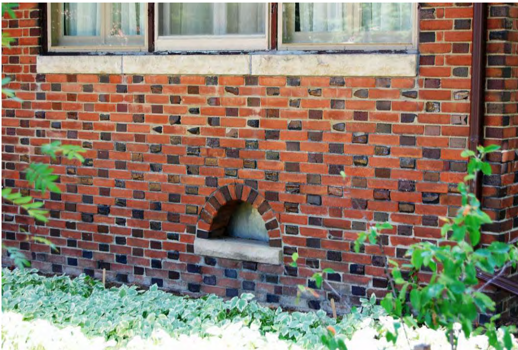
Figure 6: Detail showing the scupper below what might once have been an open porch at the corner of the house near the intersection of Isabella Street and Lorne Avenue. The photo also shows the stone sills found under most structural openings.
