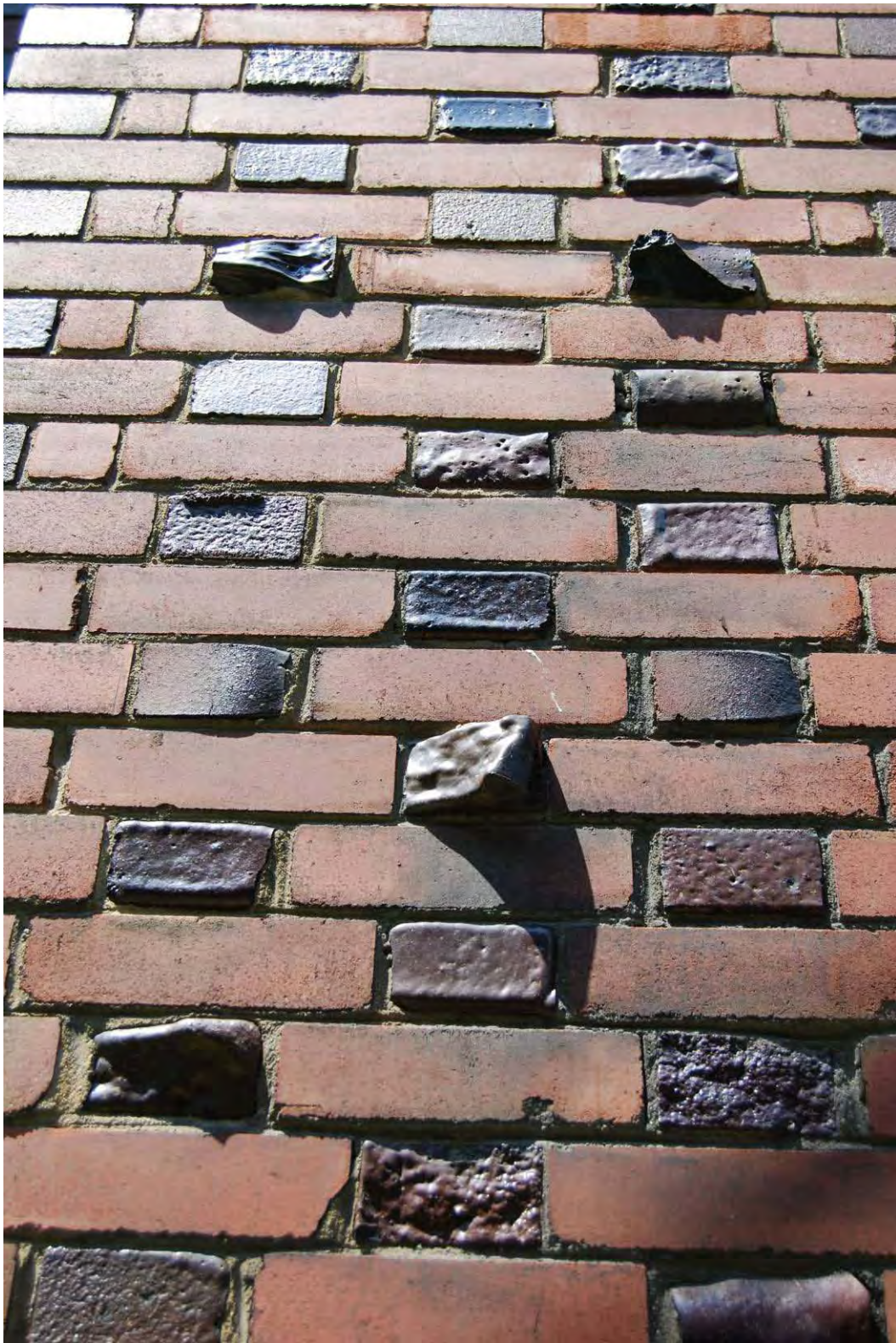
Figure 10: Detail of chimney stack on south elevation showing the unusual use of clinker brick, and oddly shaped specials laid in a contrasting pattern against a background of Brampton hard pressed brick.
