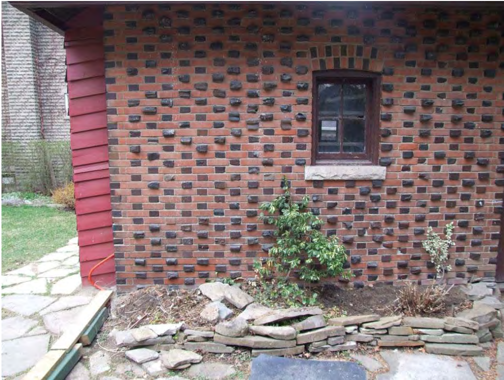
Figures 13 and 14: Detail photos showing portions of the detached garage located at the south-east corner of the rear yard. The original structure exhibits the same unique masonry patterning and texture as the main house. (photos by current owners).
