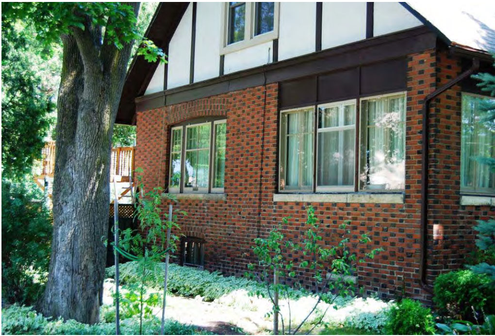
Figure 5: Detail showing a portion of north elevation and banks of wood sash windows.
