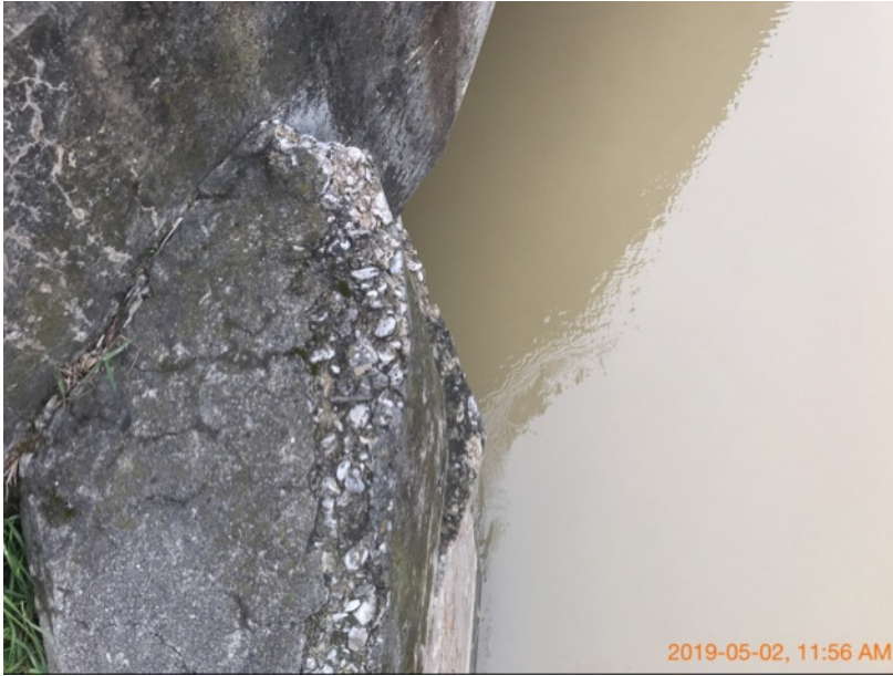
Honeycombing in top of southeast retaining wall.
