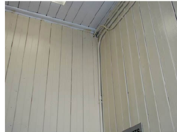
Detail of beaded tongue in groove wood paneling on walls and ceiling in main hallways. (east entrance).
