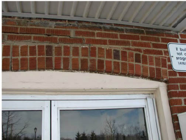
Detail showing portion of masonry wall on front façade. This image shows the brick arch of the east entrance. Note step crack. Masonry repairs are required.
