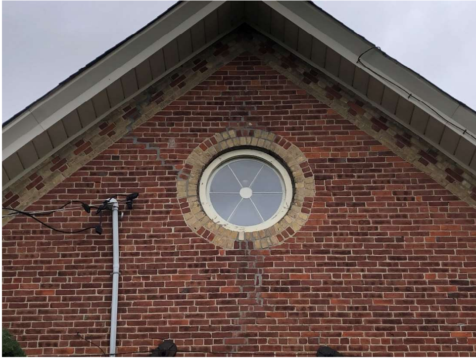
Image 2: Detail of the bullseye window and dichromatic brick pattern under the gable eaves.
