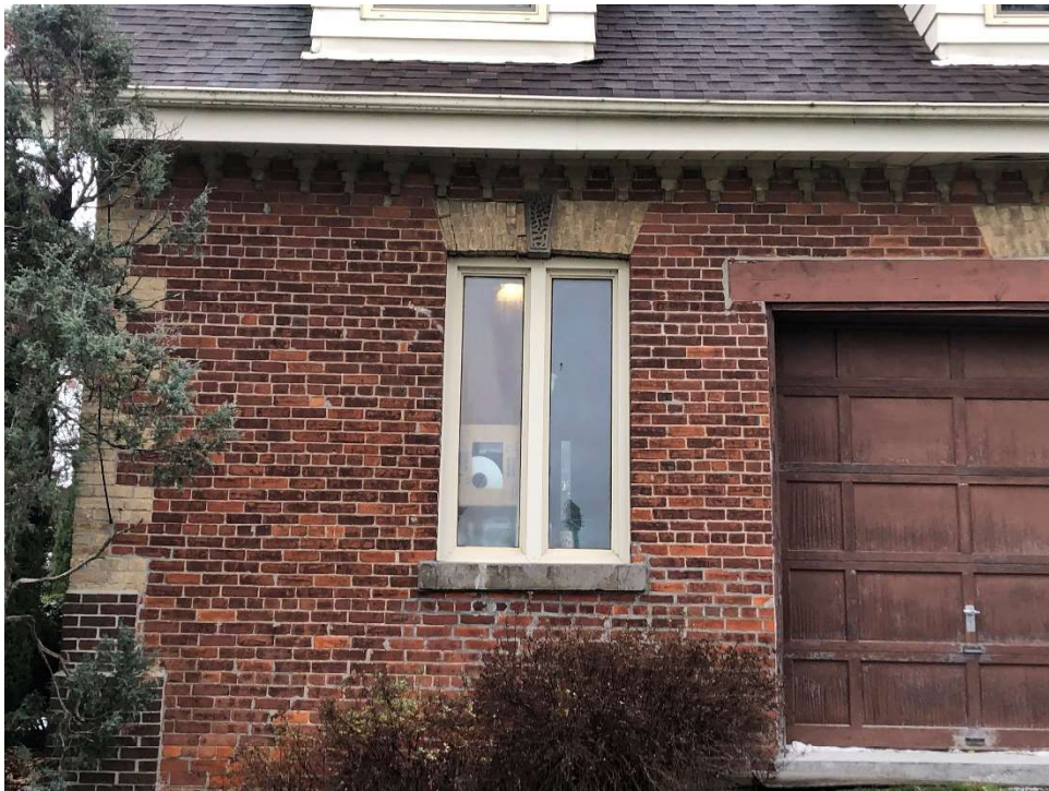
Image 6: View of a window opening on the north elevation of the schoolhouse.
