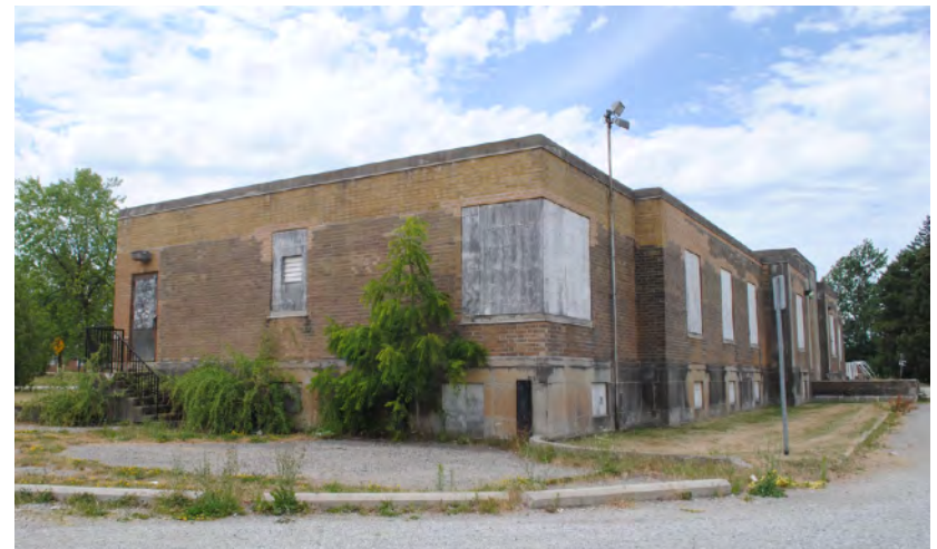
Figure 5: The 1938 Administration Building, designed by James Henry Craig, notable for its Modern Classicism style, which remains rare in Brampton. Images: GBCA.
