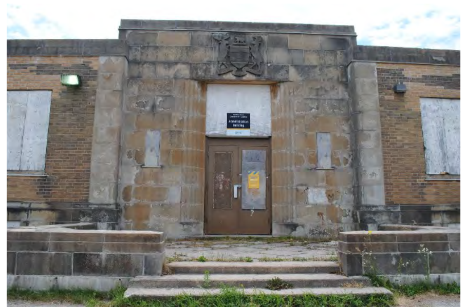
View of the main entrance to the former OPP Administrative building. The entrance features fluted pilasters flanking the recessed entrance, with a large, square transom. The Coat of Arms for the Province of Ontario rendered in cast concrete is visible over the double leaf wooden doors. The building is currently vacant.
