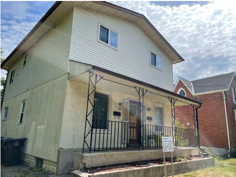
1920s 'QUARRY FACED' CONCRETE BLOCK FOUNDATION – WITH LATER STUCCO AND VINYL CLADDING ABOVE (2 ND FLOOR IS LIKELY AN ADDITION) – VINYL WINDOWS OF VARIOUS SIZES – MODERN CONCRETE STOOP AND PORCH WITH IRON RAILING & POSTS
