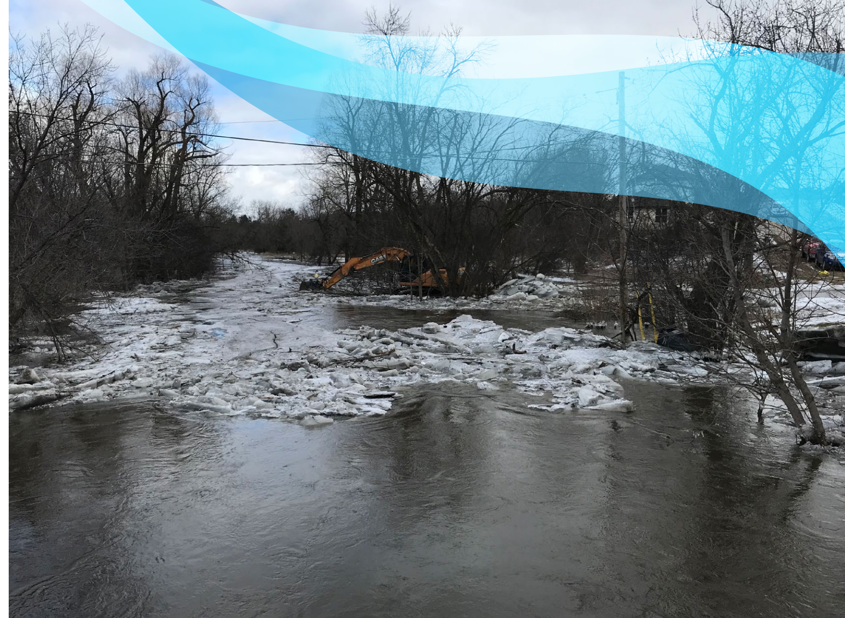
Mechanical Ice removal at an ice jam in the Humber River, downtown Bolton, March 16, 2019. Photo credit : Toronto and Region Conservation Authority
