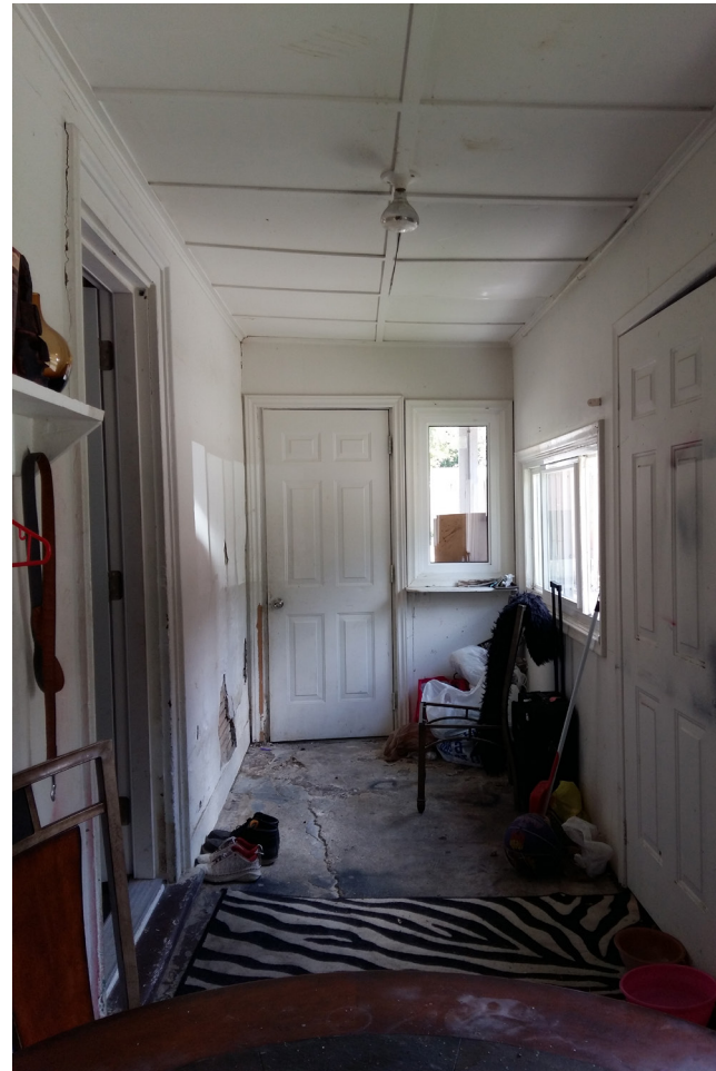
Cheaply constructed sun room added onto the rear additions.
