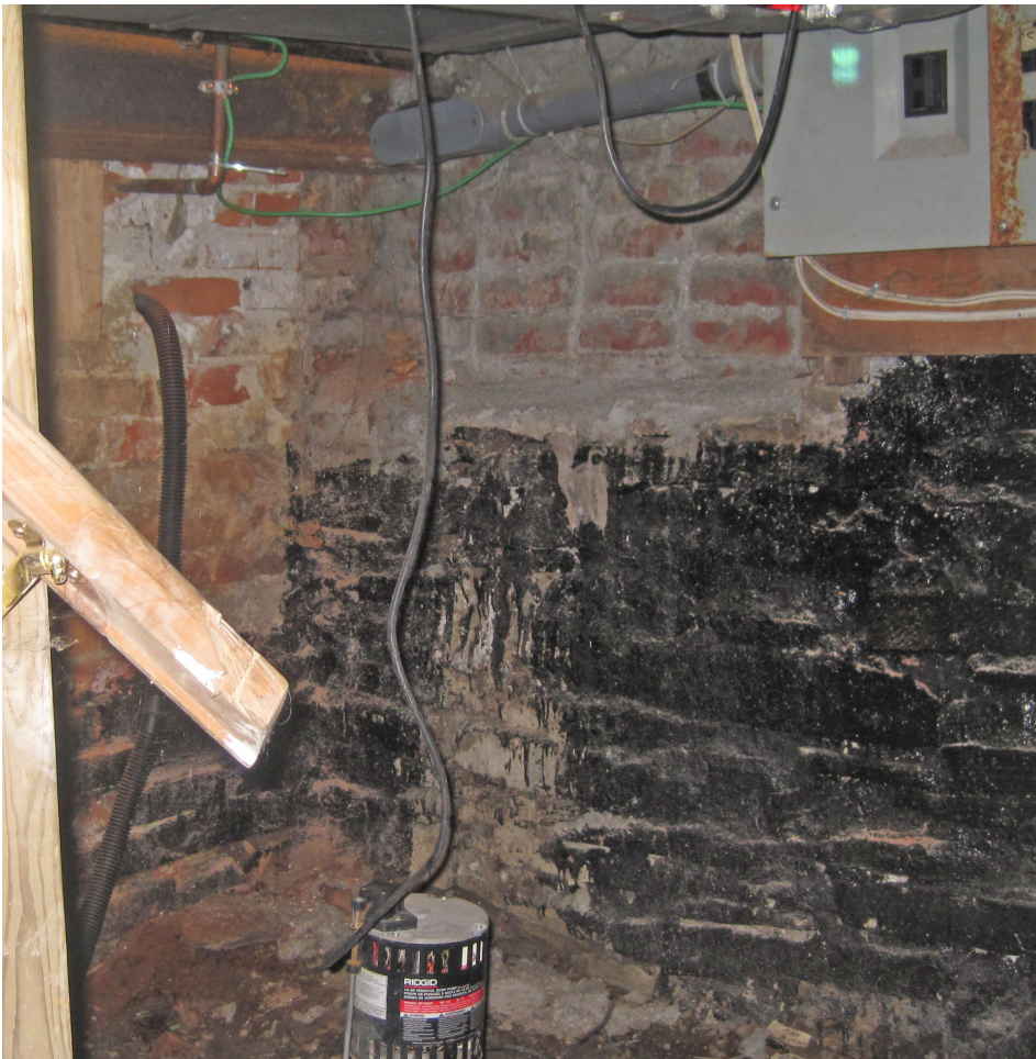
Walls are of brick masonry construction. There is some deterioration of the brick occurring.
