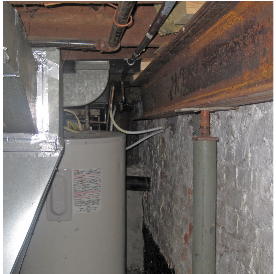
A steel beam supported by steel jacks is located against the south wall. As in the basement of 164 the beam does not run the entire length of the basement.
