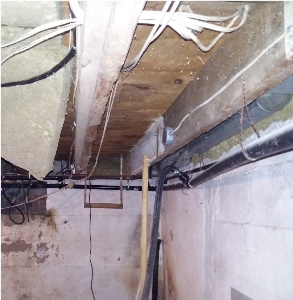
The joists in the basement of 164 have been doubled up. This appears to have been done in response to the rot that has set into what were presumably the original joists.
