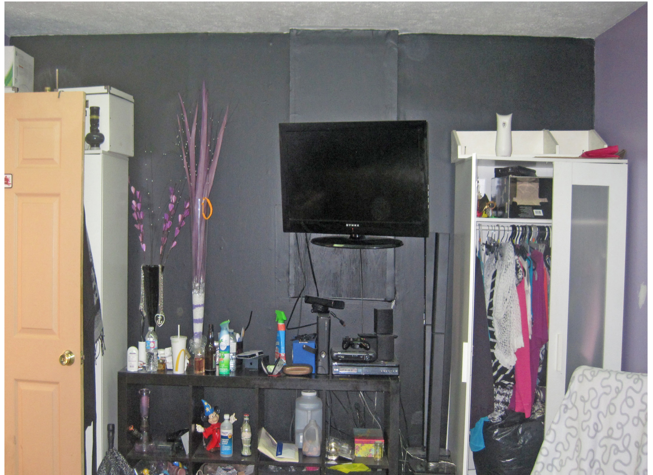
Bedroom of the ground floor unit, bump out in the wall marks location of possible duct work.
