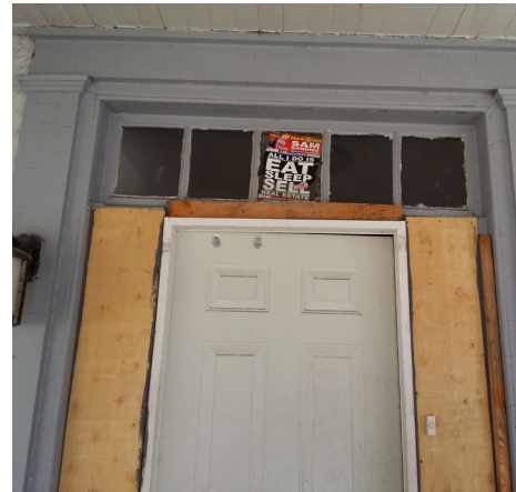
Transom and door trim remain on 164 Main though the door has been replaced and sidelights are boarded over.
