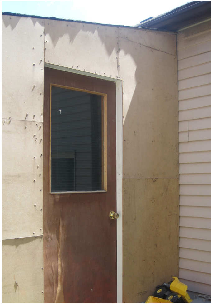
Shed structure on North side of the building, it is not original to the house.
