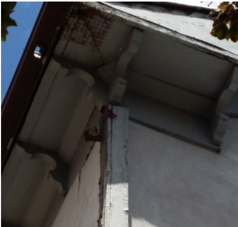
Brackets run along the soffit and deep fascia of the roof on the north, west and south sides.
