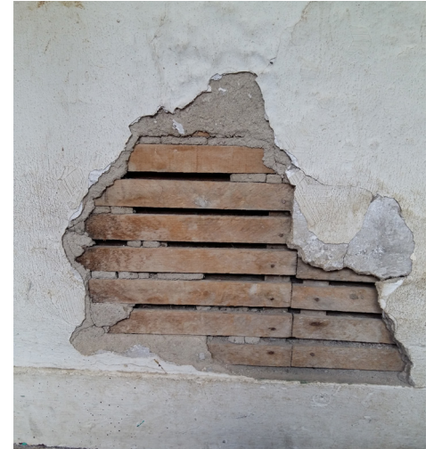
Sawn wood lath, visible in sun room of 164 on what would have been the exterior wall of the original building.
