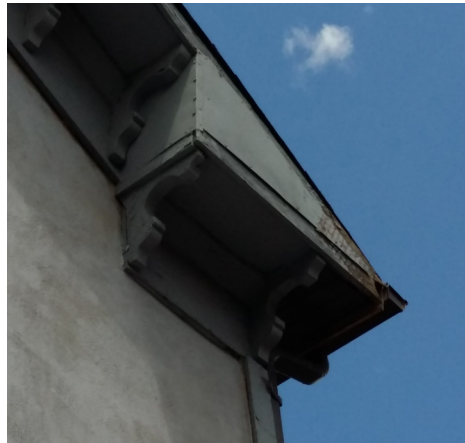
Gable ends have returns at the corners which are supported by brackets.
