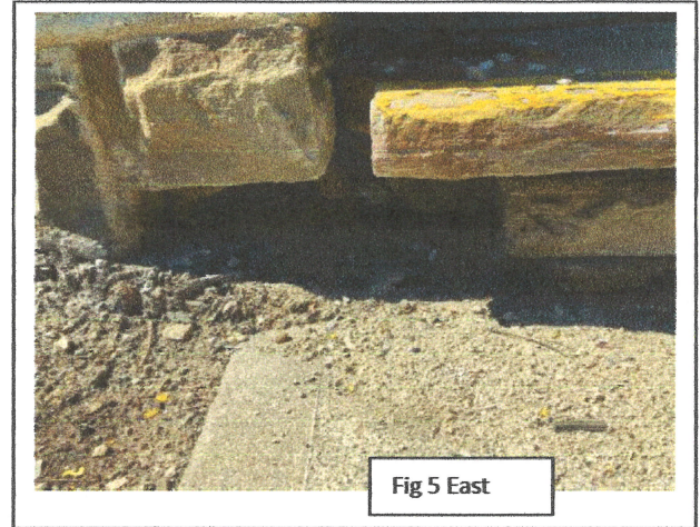
Missing Vertical support at ground level.
