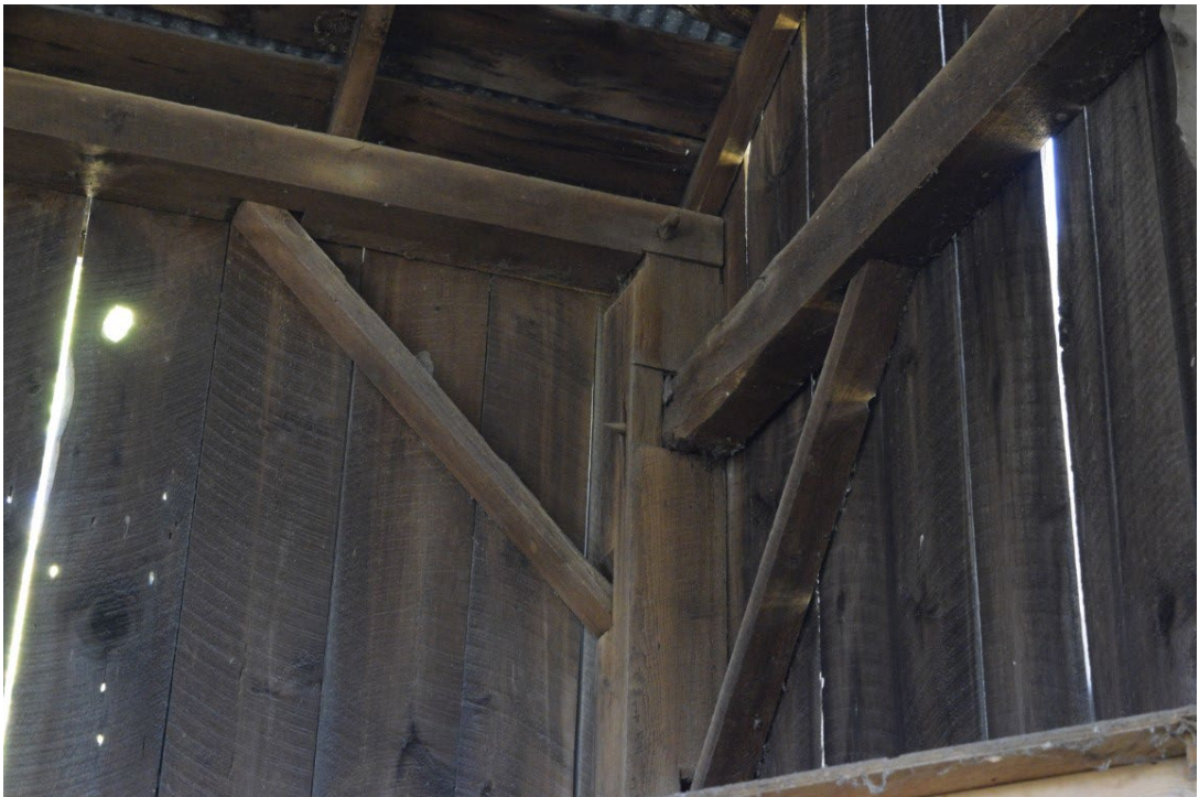
Figure 61: Typical timber framing utilizing wooden pegs and circular sawn timbers and braces
