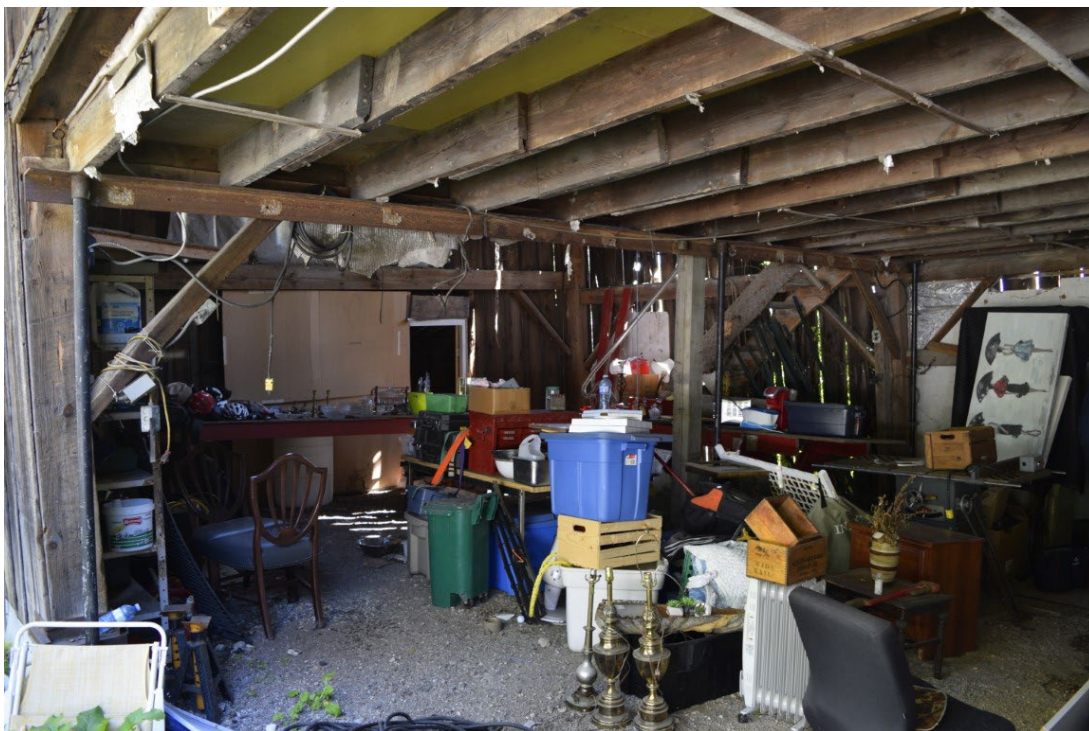
Figure 59: First floor of outbuilding, partial second floor is a later addition constructed of modern dimensional lumber
