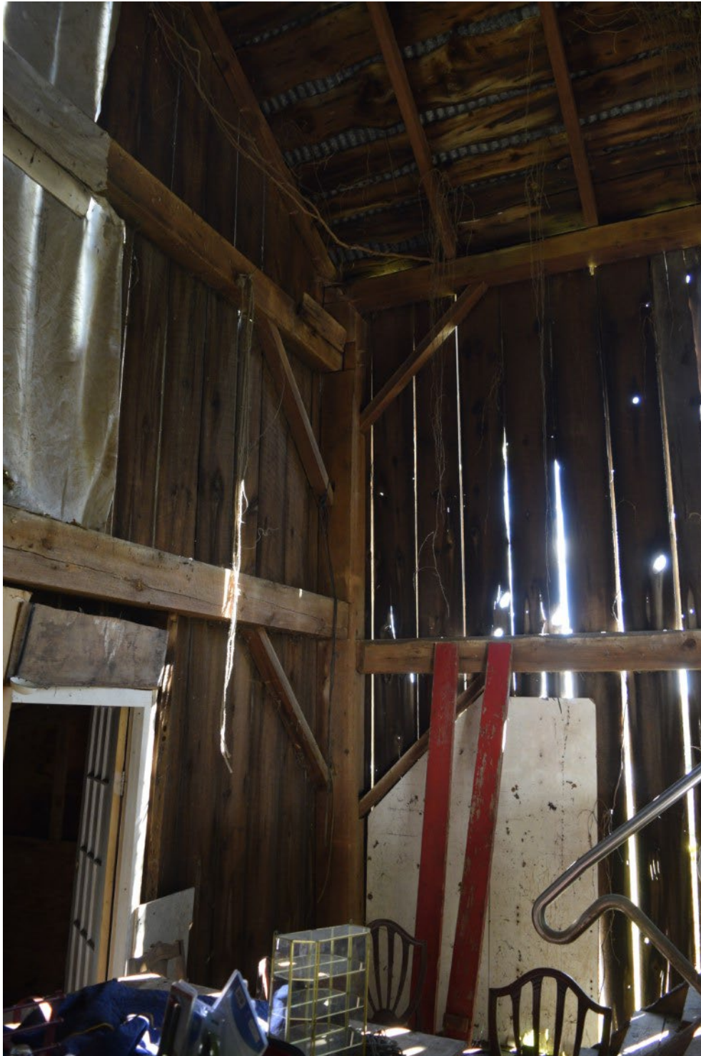
Figure 62: Representative depiction of outbuilding construction
