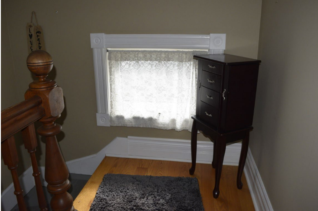
Figure 30: Example of original baseboard and window trim second floor of front apartment, note original newel post
