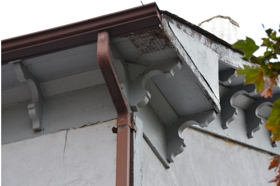
Figure 11: Original wood soffit, frieze board, brackets and fascia, as well as return eave (Source: City of Brampton)
