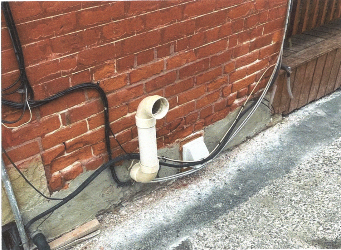
Deteriorated Brickwork and Parging above Foundation. Previous hard repointing visible
