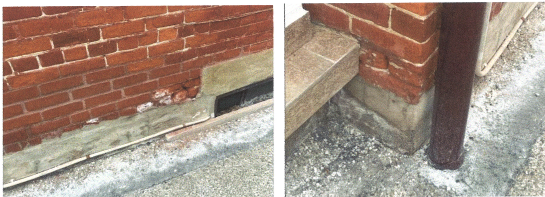
Deteriorated Masonry at Foundation and Open Joints (Typ).
