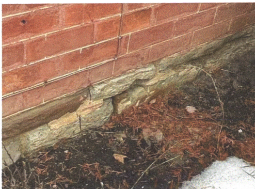
Gaps at Foundation
