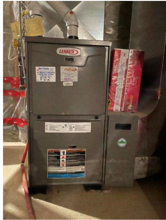
Figure 37: Log House - Furnace
