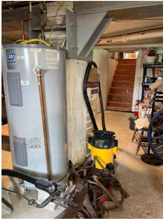
Figure 36: Main House - Hot Water Cylinder
