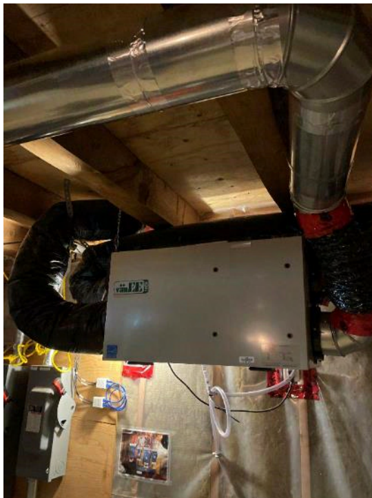
Figure 38: Log House - Air Exchange Unit
