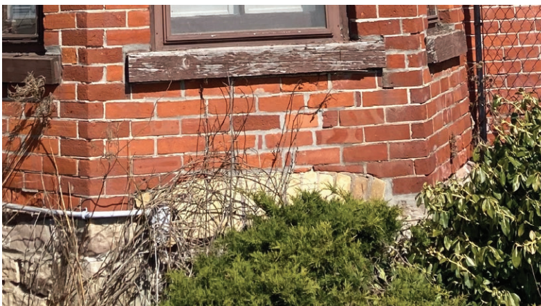
Evidence of step cracking below the bay window sill, infilled with unsympathetic mortar (ERA, 2023).
