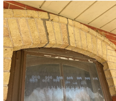
Unsympathetic pointing above the north porch window (ERA, 2023).
