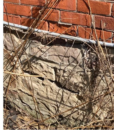
Severe deterioration of the stone foundation (ERA, 2023).
