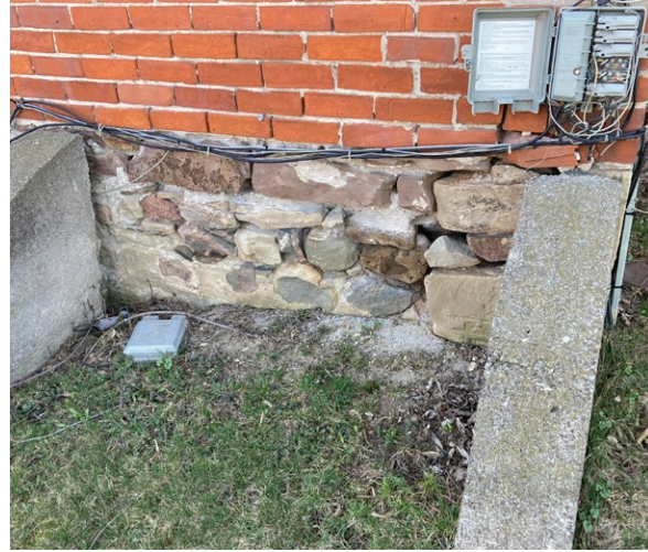
Severe deterioration of foundation pointing (ERA, 2023).
