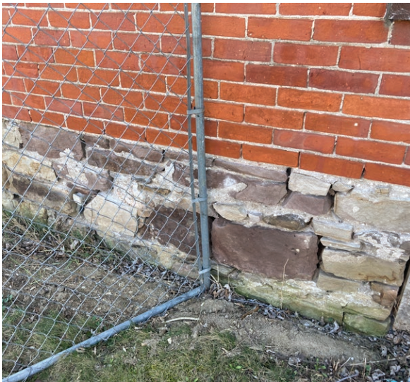
Severe deterioration of foundation pointing (ERA, 2023).
