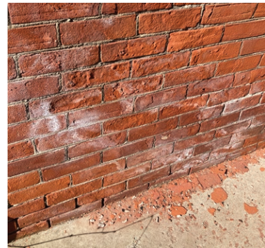
Masonry spalling on the porch level (ERA, 2023).
