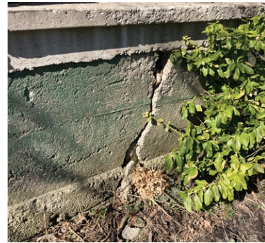
Cracking on the porch's stone foundation (ERA, 2023).
