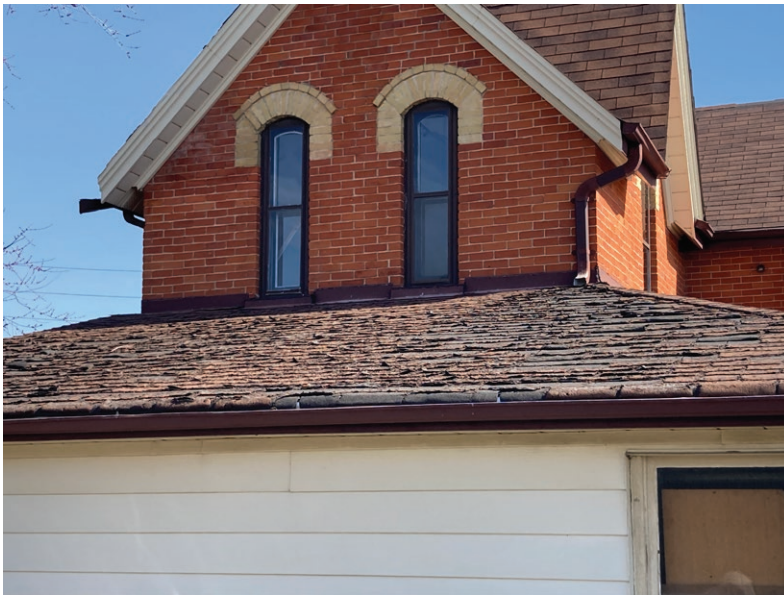
Defective shingles on the rear addition (ERA, 2023).
