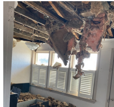
Collapsed ceiling in first floor south addition (ERA, 2023).
