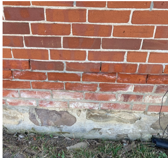
Efflorescence and spalling (ERA, 2023).
