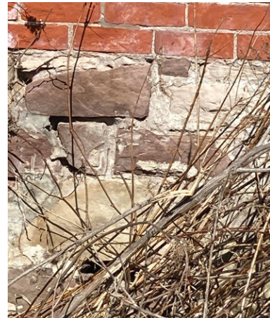
Severe deterioration of the stone foundation (ERA, 2023).
