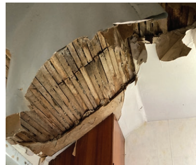
Collapsed ceiling in the second floor bathroom (ERA, 2023).
