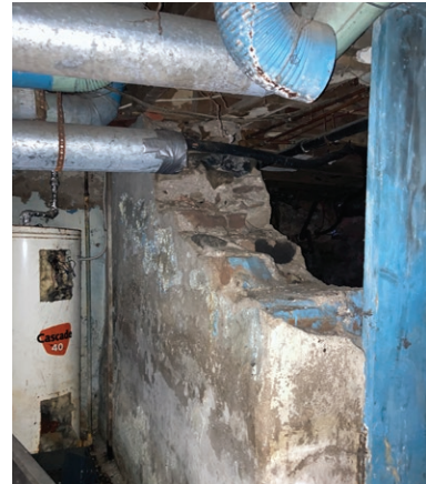
Damaged rubble foundation wall (ERA, 2023).
